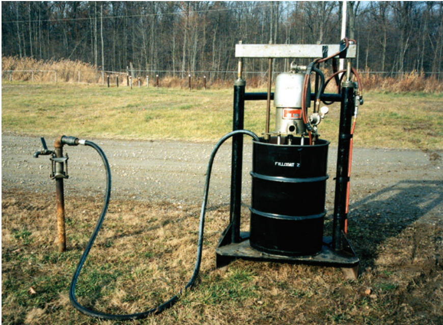
Fill-Coat #2 being pumped by air-driven mastic pump from 55-gallon drums into the casing vent.
